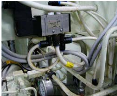
point; hose joint 59. 4L/min
