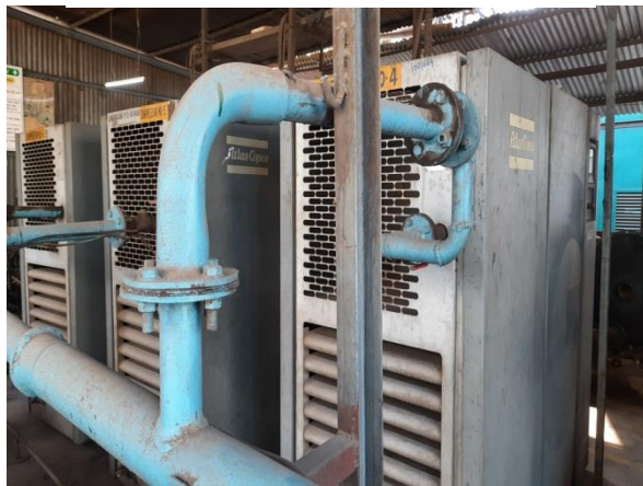
Air compressors at Paranjape Autocast
